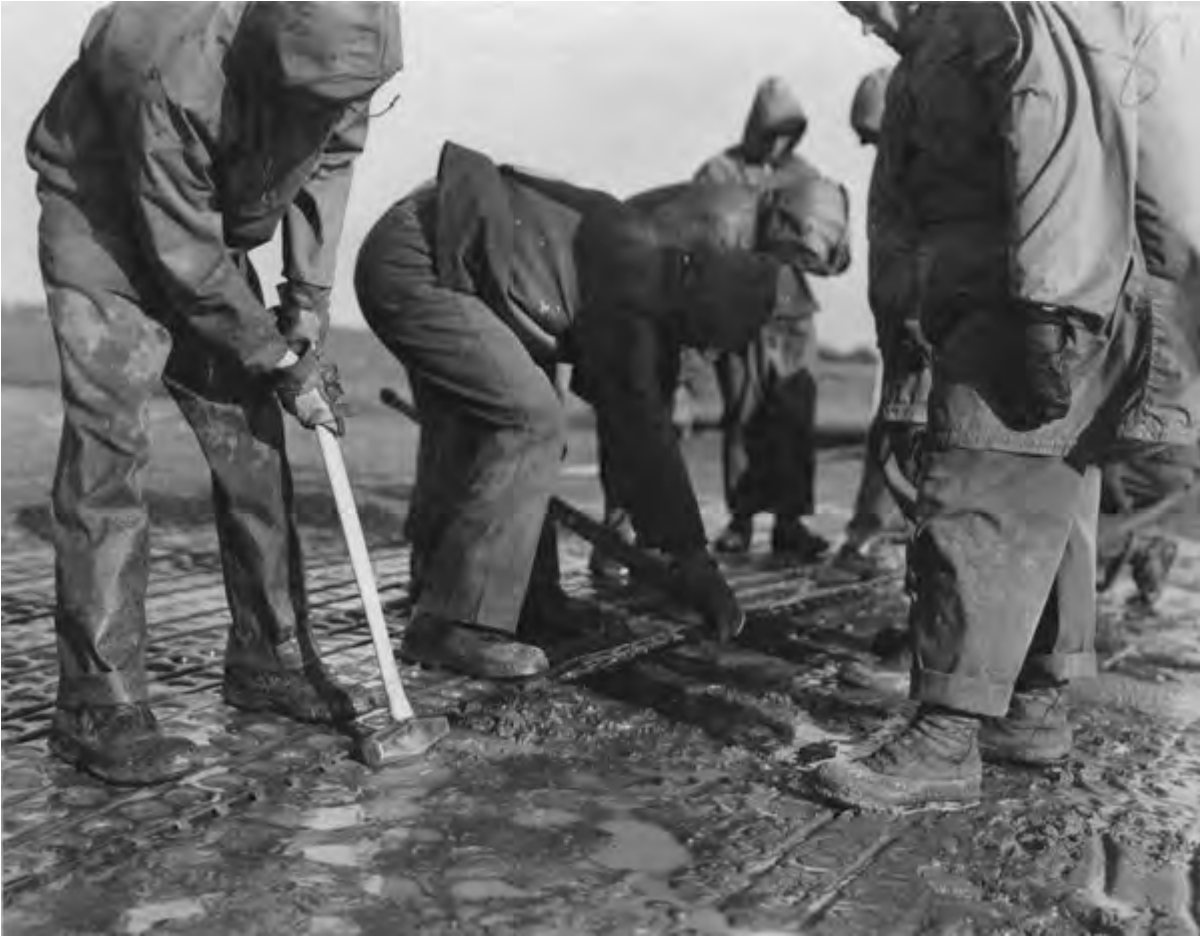
Each section of mat ran 10 feet long by 15 inches wide, with integrated hooks and slots so a construction battalion of Navy "SeaBees" could knock together a 3,000-foot runway with only a sledgehammer. This crew is seen on Amchitka Island in the Aleutians in 1943. (NARA)
