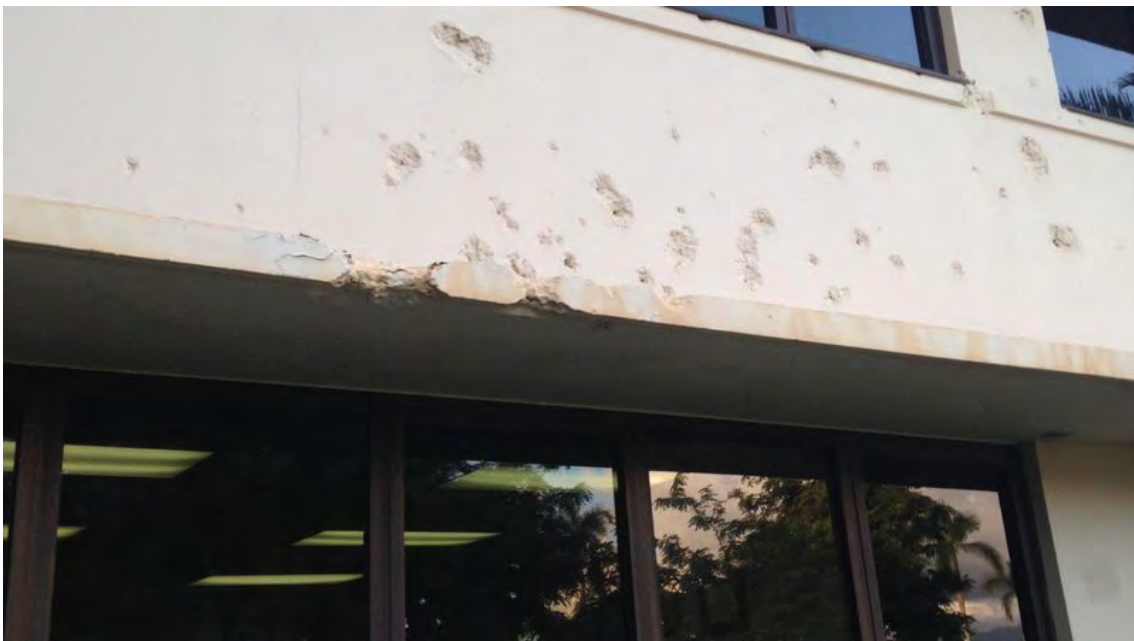
The exterior of PACAF headquarters is still pocked with bullet holes. (John Sotham)
